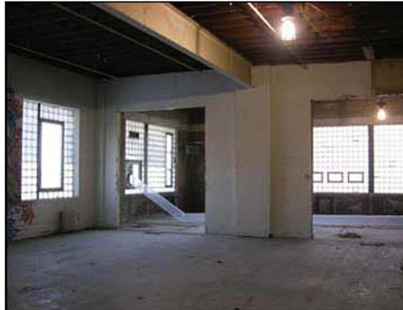
Hillcrest Development transformed a polluted, 5.6-acre former heavy industrial site in northeast Minneapolis into Crown Center, which will house a variety of professional, industrial, medical and creative businesses. Shown here is one of the buildings before the clean-up and renovation. Grants to clean up the pollution on the site came from three agencies, including the Met Council.
